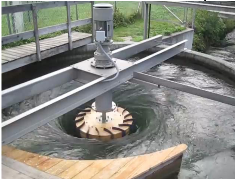
ZOTLÖTERER - worldwide first Gravitation Water Vortex Power Plant https://www.youtube.com/watch?v=oo_mP18IXMo
